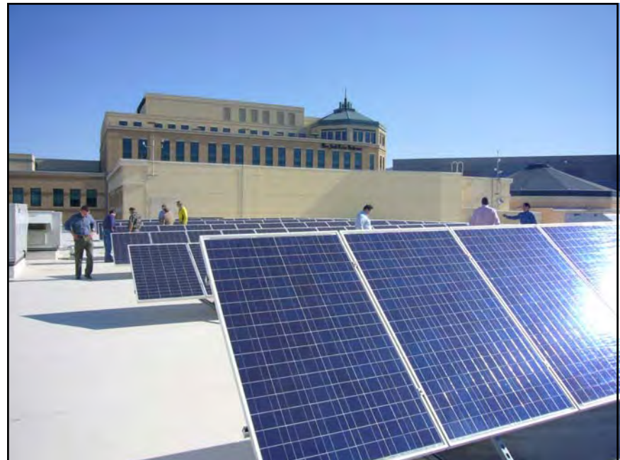
A solar array at the Gateway development in Salt Lake City.
